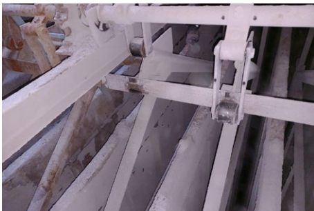
Coromax is compatible with any type of ESP. Here, an installation with tumbling hammers.
