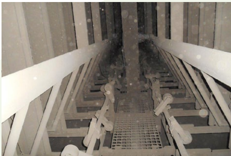
ESPs of any layout/footprint can be upgraded with Coromax. This upgraded installation features a rapping system with adjacent gangway.
